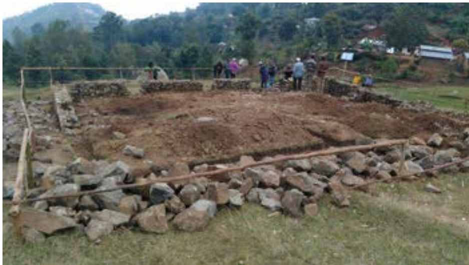
..... Photo 3. Foundation of a health facility being built in a T4D village in Tanzania.
